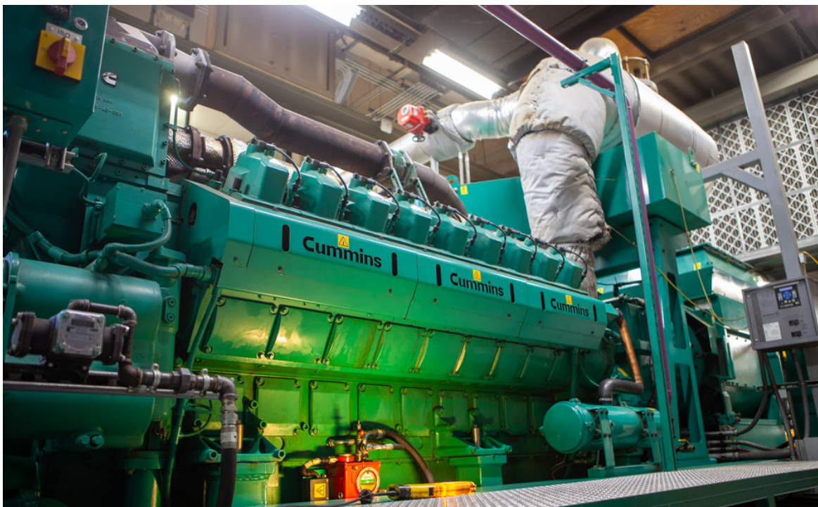
The 18-cylinder 2000 kW Cummins cogeneration engine.
