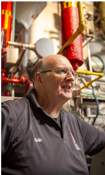
Bob with Boiler Number One.
