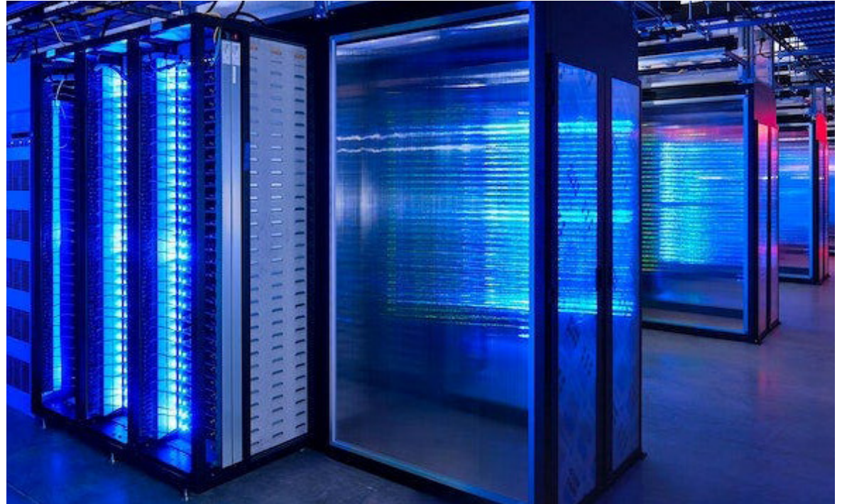
A server room. Licensed for use by Creative Commons.
